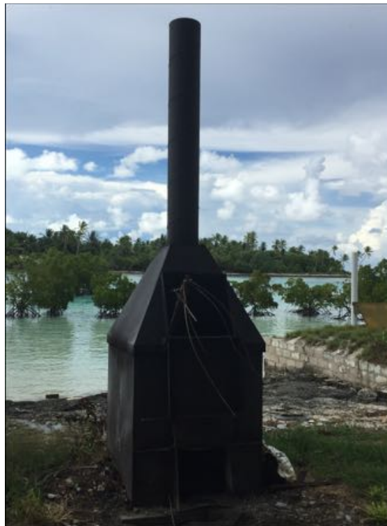
Photo 17 – Quarantine Waste Incinerator
