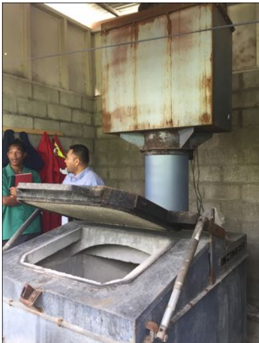
Photo 14 – Recently Installed Incinerator
