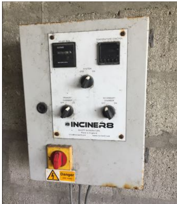
Photo 15 – Corroded Control Panel
